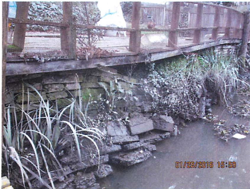
A closer view of the eroded rock-facing. The photo was taken shortly after the low tide of the day.
