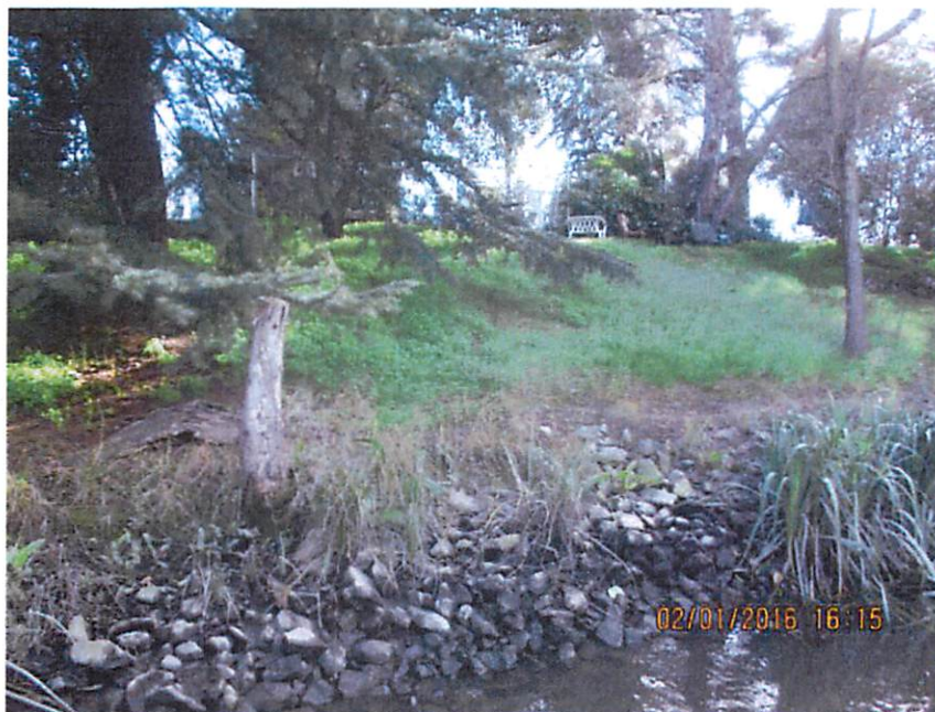
The vegetated portion of the levee embankment shown in the photo, and to the right of the trees in the foreground, cracks due to lack of moisture. Recent rains have left no evidence of cracking.
