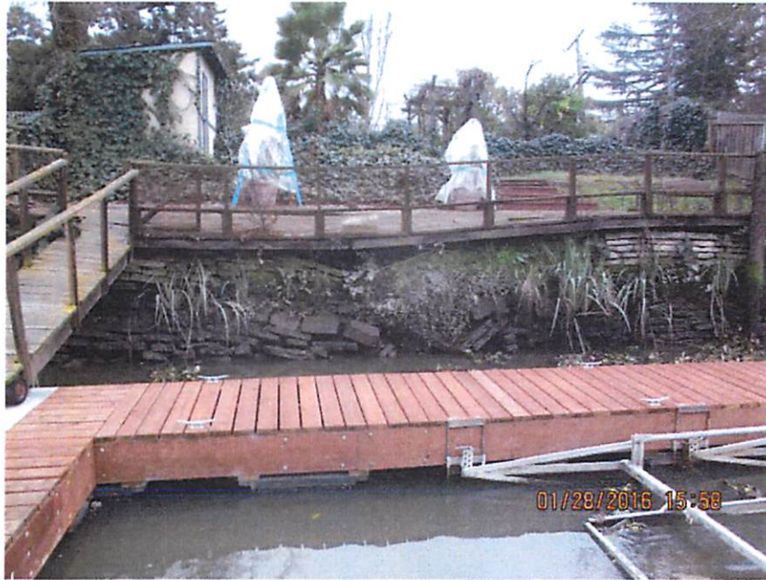
The rock facing atop the rip rap on the waterside levee of the Richenberg residence. Peering through the hole showed nothing but rip rap that appeared to have settled due to erosion of the underlying soil. Note the sagging of the wooden deck as a consequence of the eroded rock-facing.
