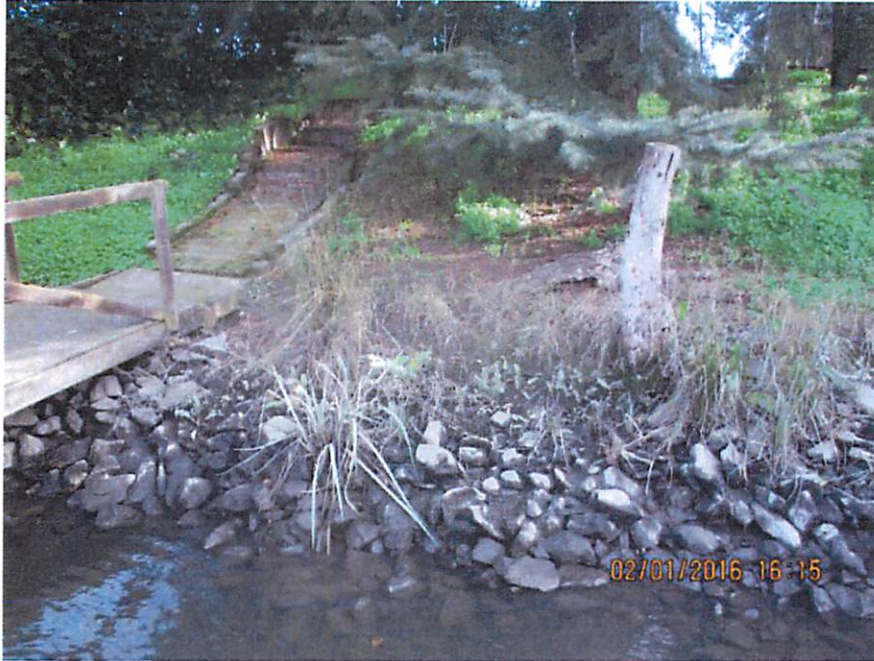
The waterside levee embankment on the Moore's property. Daniel stated that the high tide reaches the foot of the wooden gangway upslope from the rip rap.
