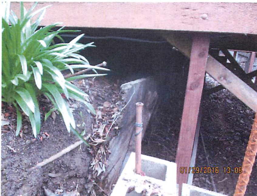
The levee crown appeared to be at the same elevation as the neighbors on both sides of the property in question. However, inspection revealed this 'retaining wall' about 3-feet from the crown along the entire property width.
