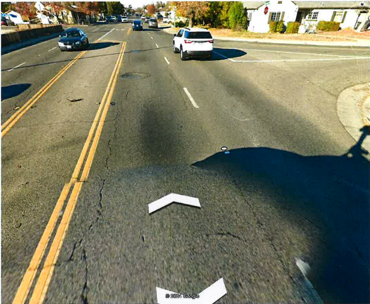
Manhole 5 is where the sewer bypass pumping returns to the system.
