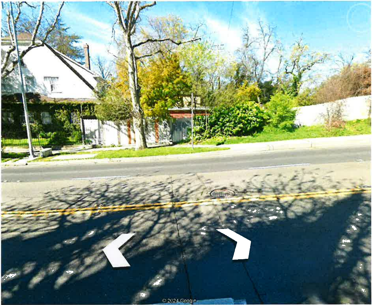
Manhole 2 is the middle of the three manholes south of the Pershing Ave. bridge.
